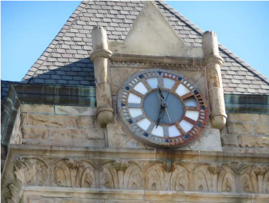
Rusted face of clock
