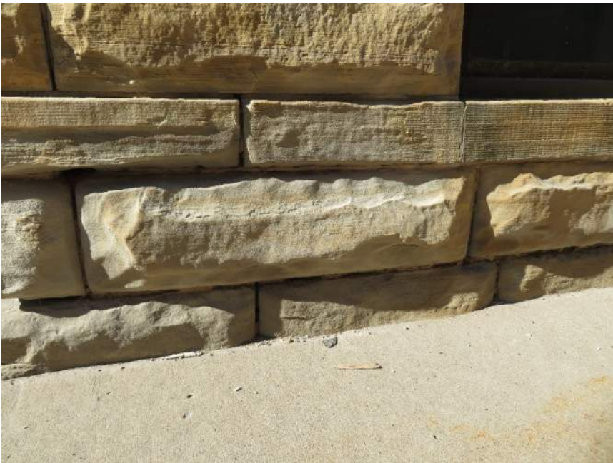
Deteriorated sandstone and mortar joints
