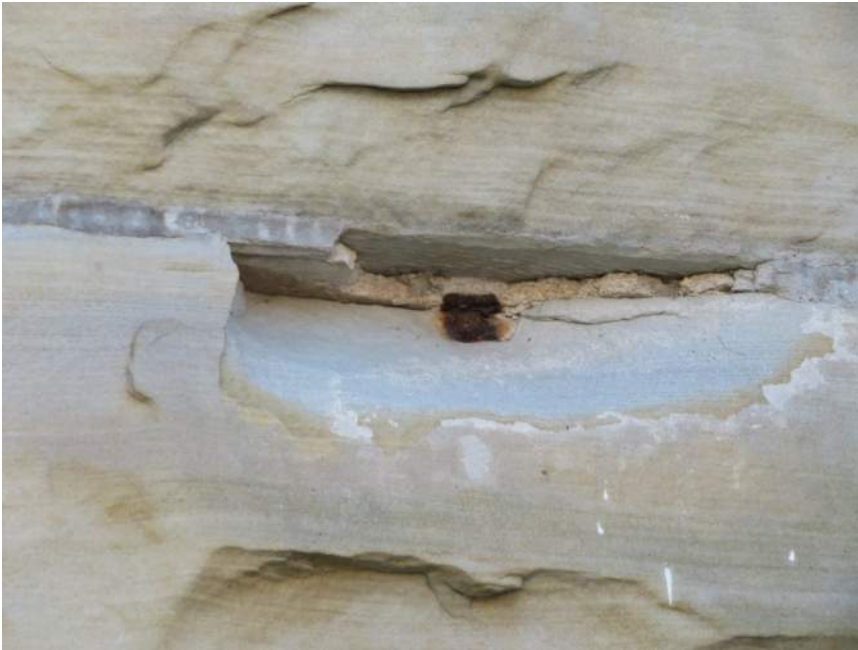
Rusted stone anchors
