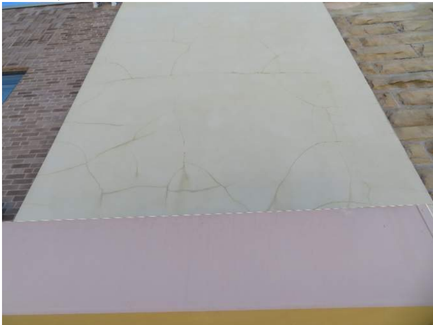
Cracks in EFIS
