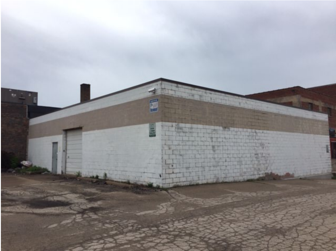
Photo #9. West (left) and south (right) elevations of Addition looking SE, shot 05-15-22.
